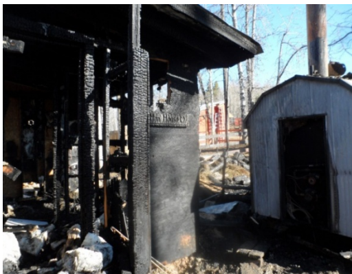
vi. After the fire
